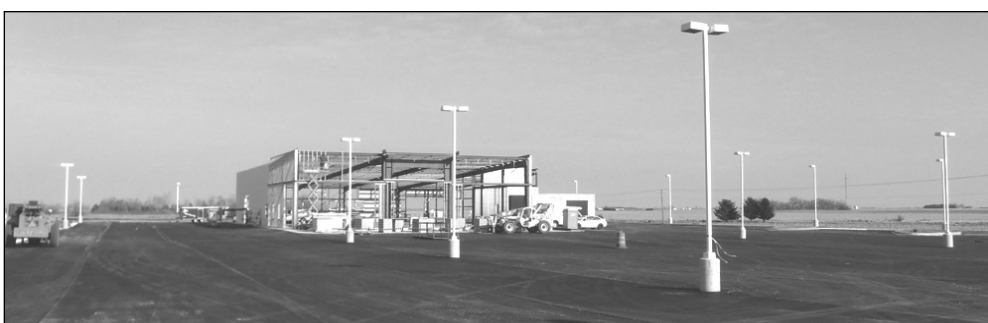
WORK ON THE NEW COUNTRY CHEVROLET facility on Route 115, on the north edge of Herscher, is progressing quickly. Asphalt was put on the lot last week, and the building is starting to go up.
