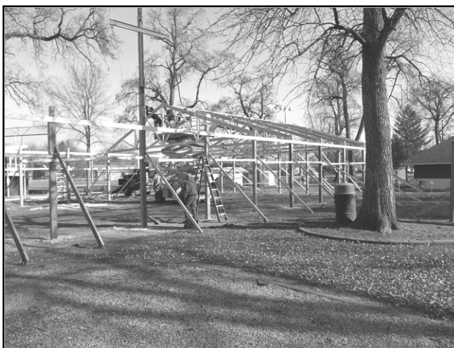
HERSCHER is putting up a large covered pavilion in Village Park, near the "big stand," and over the concrete slab that had basketball hoops at each end. The pavilion will be 45x75 feet.
