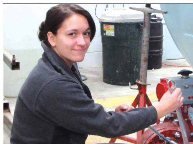
Alexa Serafinn, a fourth year apprentice, at work on the Chatsworth Water Project.
