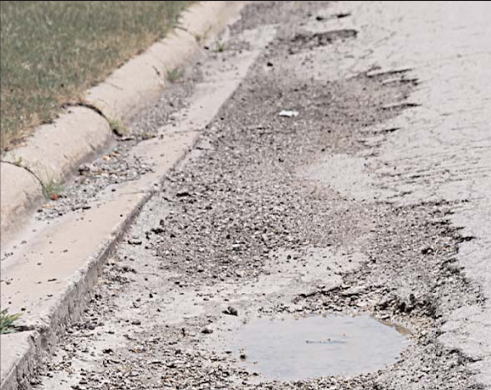
ROAD CRUMBLING on South Chicago Street in Dwight.
