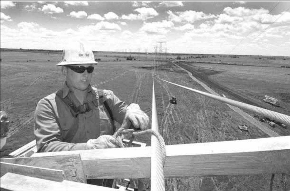
TYLER NANSTAD, a ComEd overhead lineman, goes airborne last week while working on one of the nine transmission towers between Streator and Dwight that were severely damaged by the June 5 tornado. He is among 50 ComEd employees working around the clock to build five new towers, repair others and re-string 34 miles of transmission line. No customers are affected by this work, which should continue for several weeks. Photo courtesy ComEd
