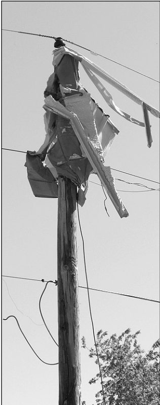
DEBRIS WRAPPED AROUND a damaged utility pole on Sunset Drive near Wilmac Street.
