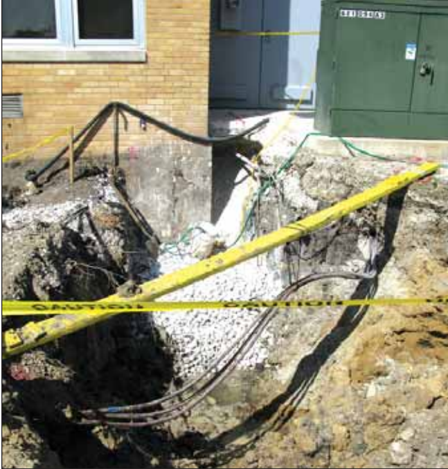
A TRENCH-TURNED-SINK HOLE caused a power outage at Dwight Township High School Tuesday, March 30, when a trench wall collapsed and pulled ComEd wires (seen under the yellow board) from a transformer (top right). Construction crews came across the unstable ground during the ongoing cafeteria expansion project.
